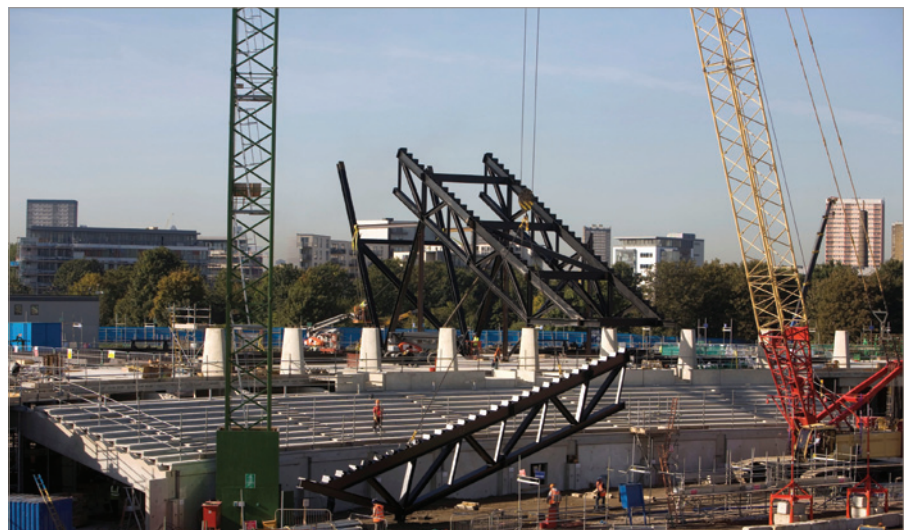
Figure 4. Prefabricated sections of upper tier steelwork during erection – setting out was refined to ensure maximum repetition of components
